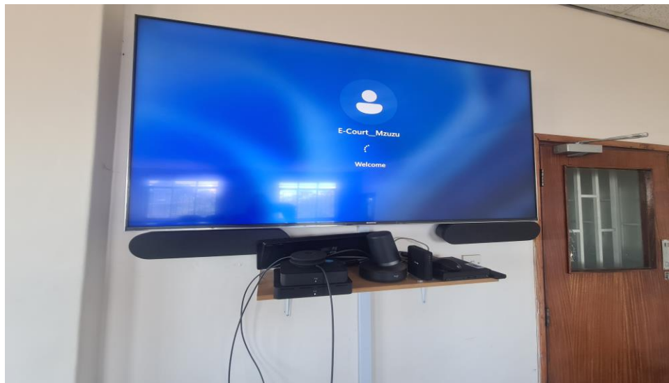
A Video Conference Facility Installed at CRM North
